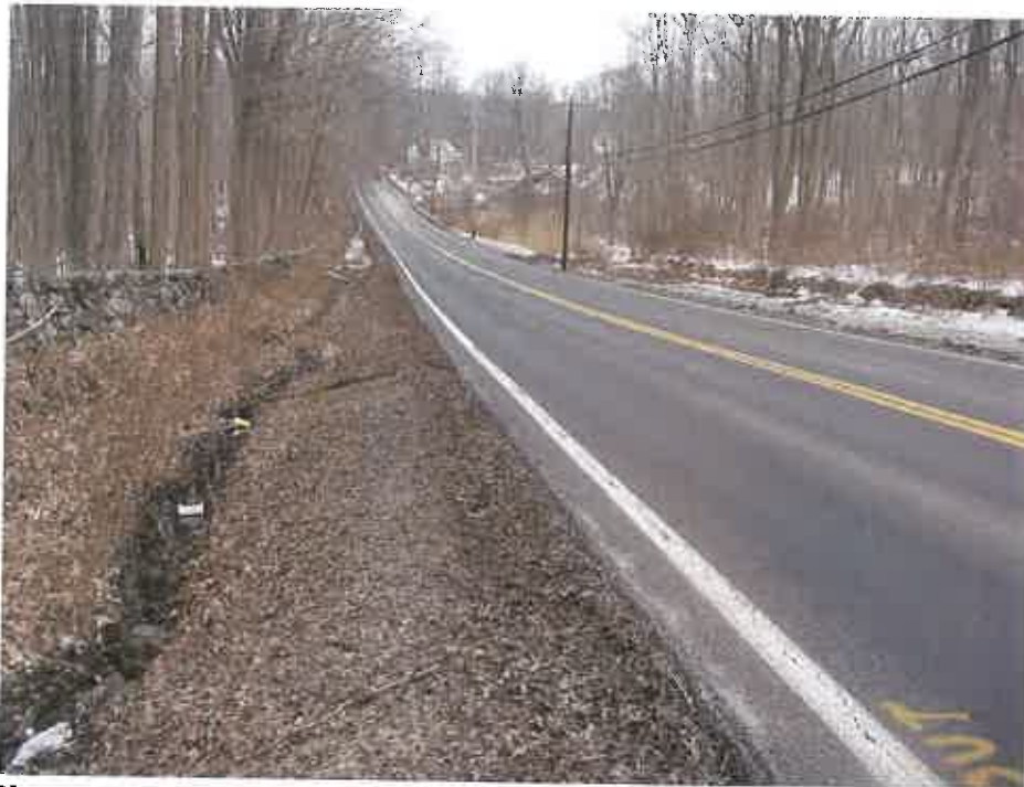
Photograph 1: Drewville Road and existing drainage ditch. View is to the east/northeast. Photograph taken February 2009.
