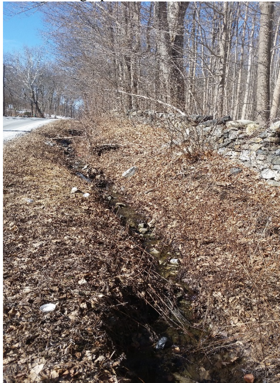
Photograph 2: Drewville Road and existing drainage ditch. View is to the west. Photograph taken March, 2015.
