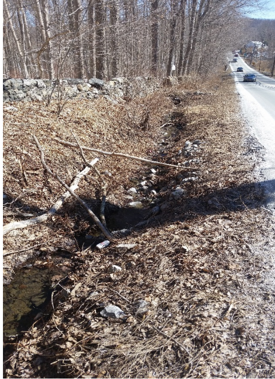
Photograph 1: Drewville Road and existing drainage ditch. View is to the east/northeast. Photograph taken March, 2015.
