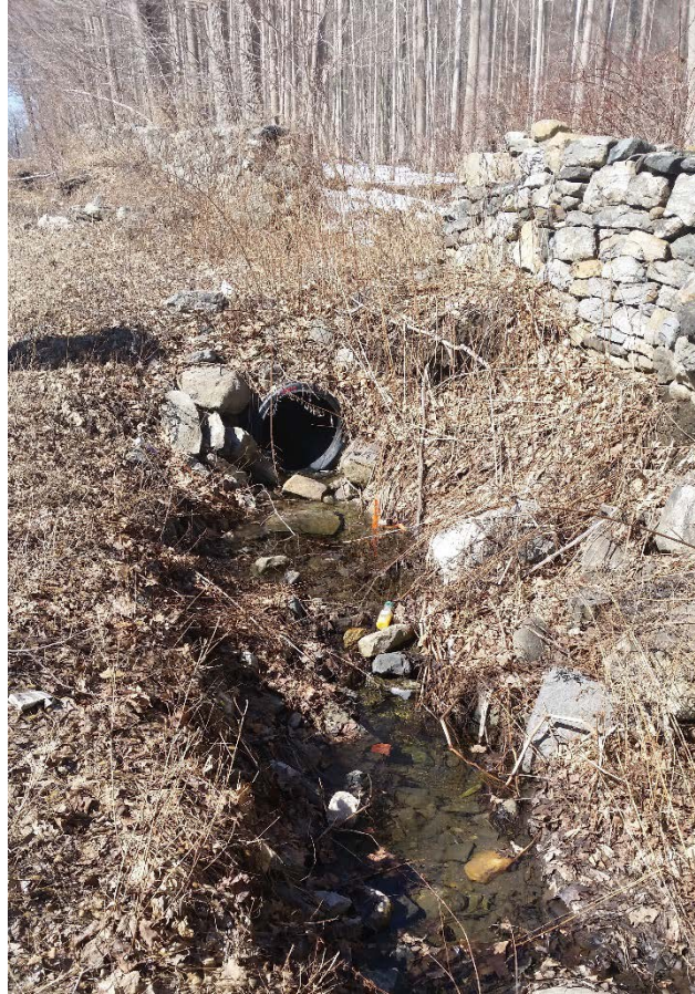
Photograph 3: Existing grass road opening in stone wall and plastic pipe culvert to be replaced. Photograph taken March, 2015.
