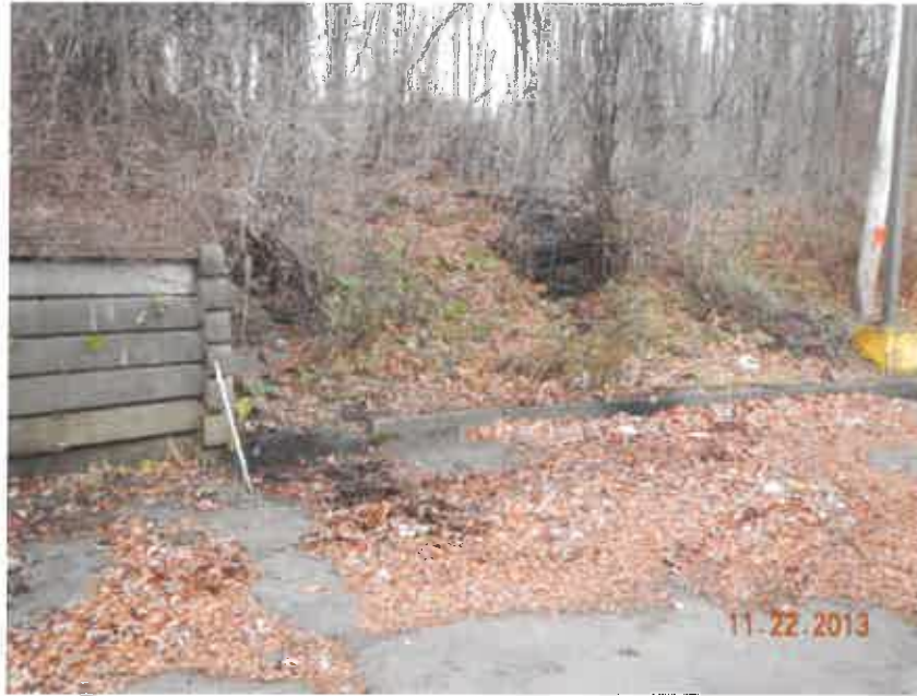
Photograph 9. Representative view of the intermittent watercourse (marked by blue ribbons) dispersing into catch basin, facing west.
