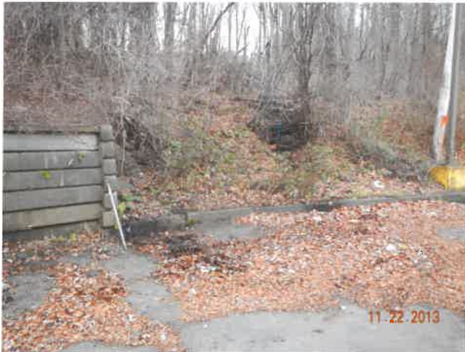
Photograph 9. Representative view of the intermittent watercourse dispersing into catch basin, facing west.
