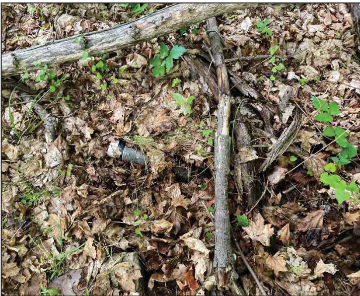
Photo 19 – Partially buried PVC pipe observed within the southwestern portion of the Subject Property
