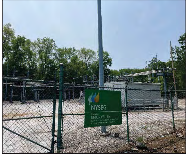
Photo 22 – View of the NYSEG Union Valley Substation located adjacent to the northeast of the Subject Property
